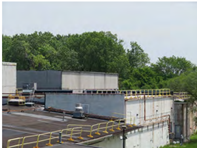
Placing bright yellow guardrails around the roof’s perimeter can be unsightly. There are ways to achieve OSHA guidelines without doing so. For instance, galvanized rails are less visually intrusive. See larger photo above.
