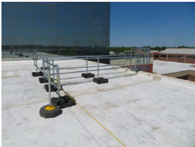
Guardrails create a walkway between a 15-foot warning line and a ladder at a roof’s edge.
