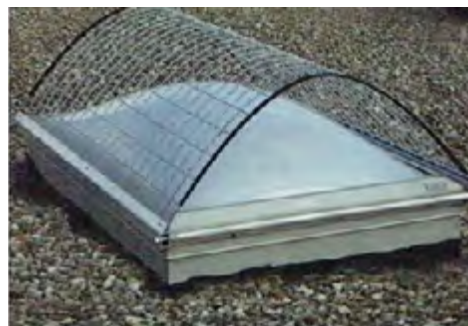
Guardrails and cages are two options for skylight safety. Frosted skylight glass prevents those on the inside from seeing the safety devices.
